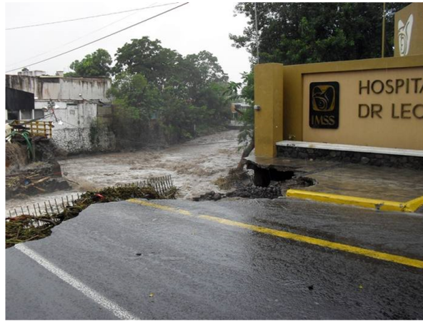
Figure 3: Damage caused to Los Maestros Avenue bridge and Dr. Leonel Ramirez general hospital during Hurricane Jova by the overflow of Colima river. (Source: El Universal newspaper, October 13, 2011)
